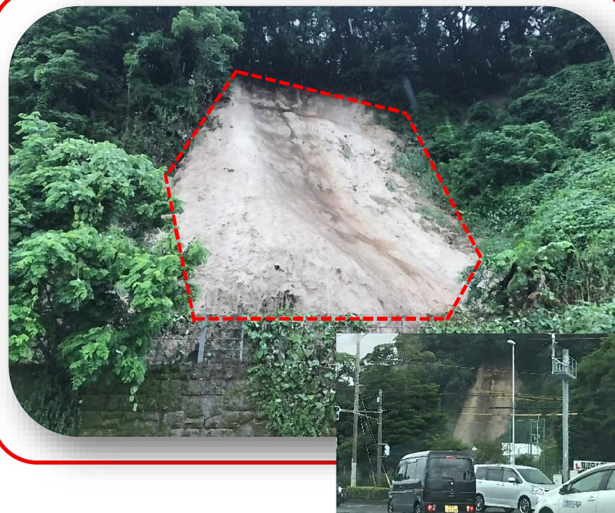
崩土発生直後(R2.7.8)
